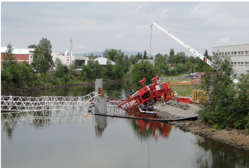
Figure 1.3: A mobile crane collapsed on a bridge construction project in Fairbanks, USA [36, CC BY 2.0]. This mobile crane lost its balance as its boom was extended beyond the permissible limit [119].
