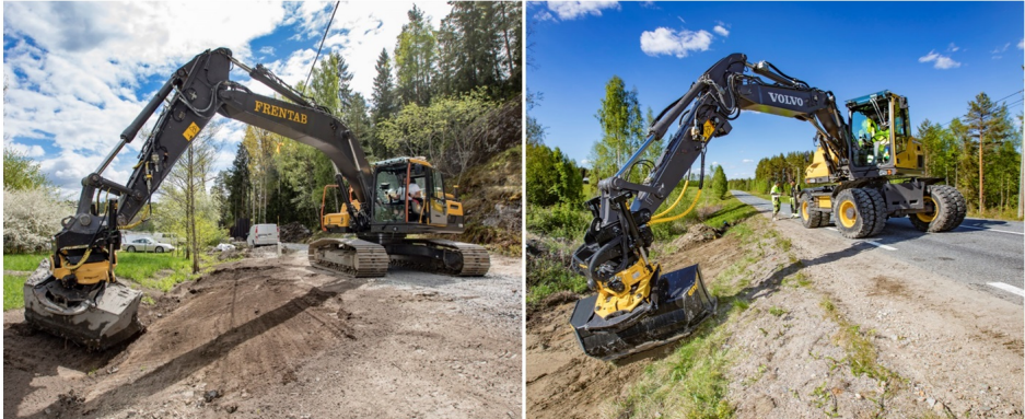
Figure 1.4: The left image shows a crawler excavator [33, CC BY 2.0], while the right image shows a wheeled excavator [34, CC BY 2.0].
